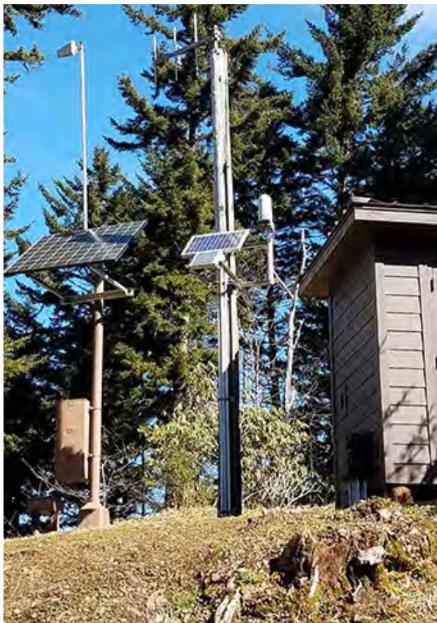
Accessory ground-mounted SES powering remote meteorological and communications equipment. Photo by Bradley Neumann.
