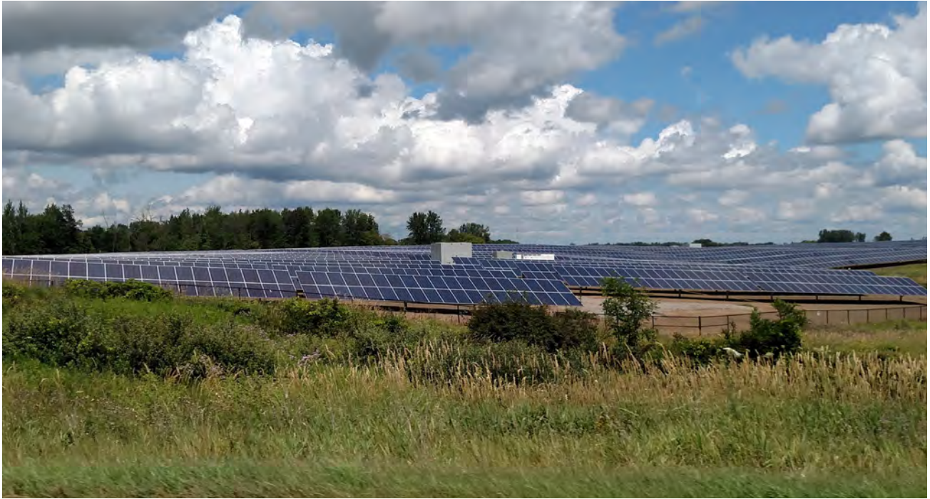
Lapeer Solar Park. Photo by Bradley Neumann.
