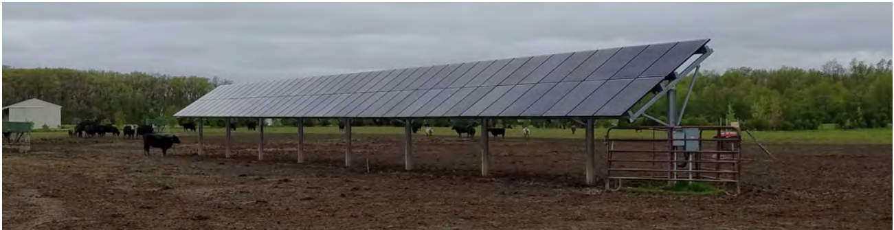
Ground-mounted SES feedlot. Photo by M.Charles Gould.
